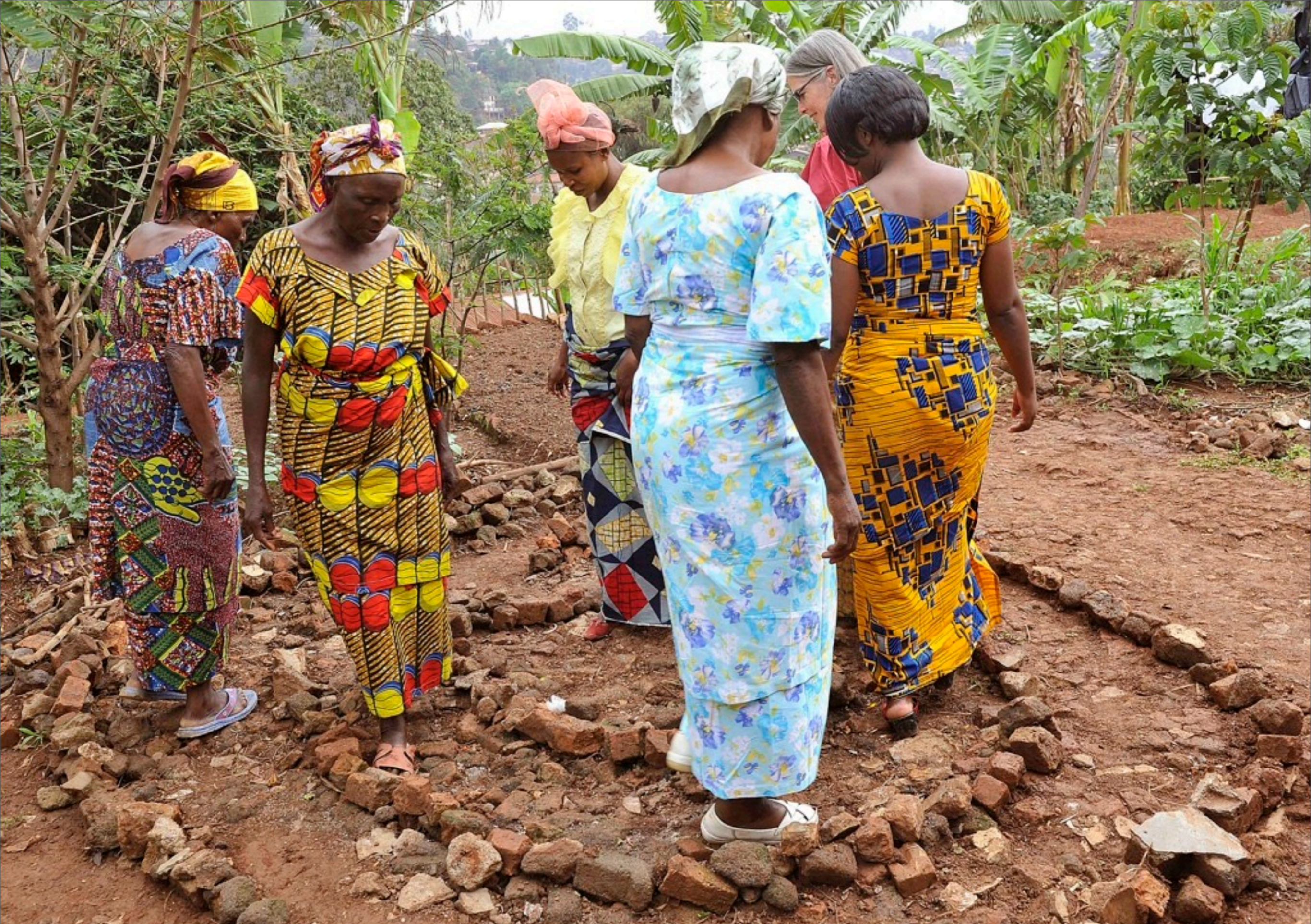
3 circuit labyrinth of earth, stone and bricks Lipandasi Home Bukavu, D. R. Congo
